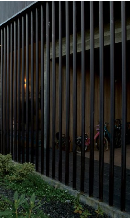
CUSTOM STEEL LOUVERS
